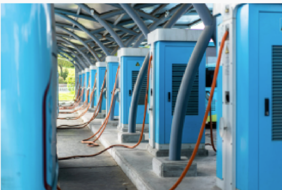
Plug-in Charging Station
